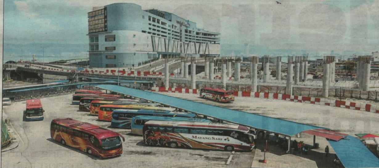
Penang Sentral terminal hub viewed from different angles (left and below) while still under construction. — Photos: LO TERN CHERN/The Star
